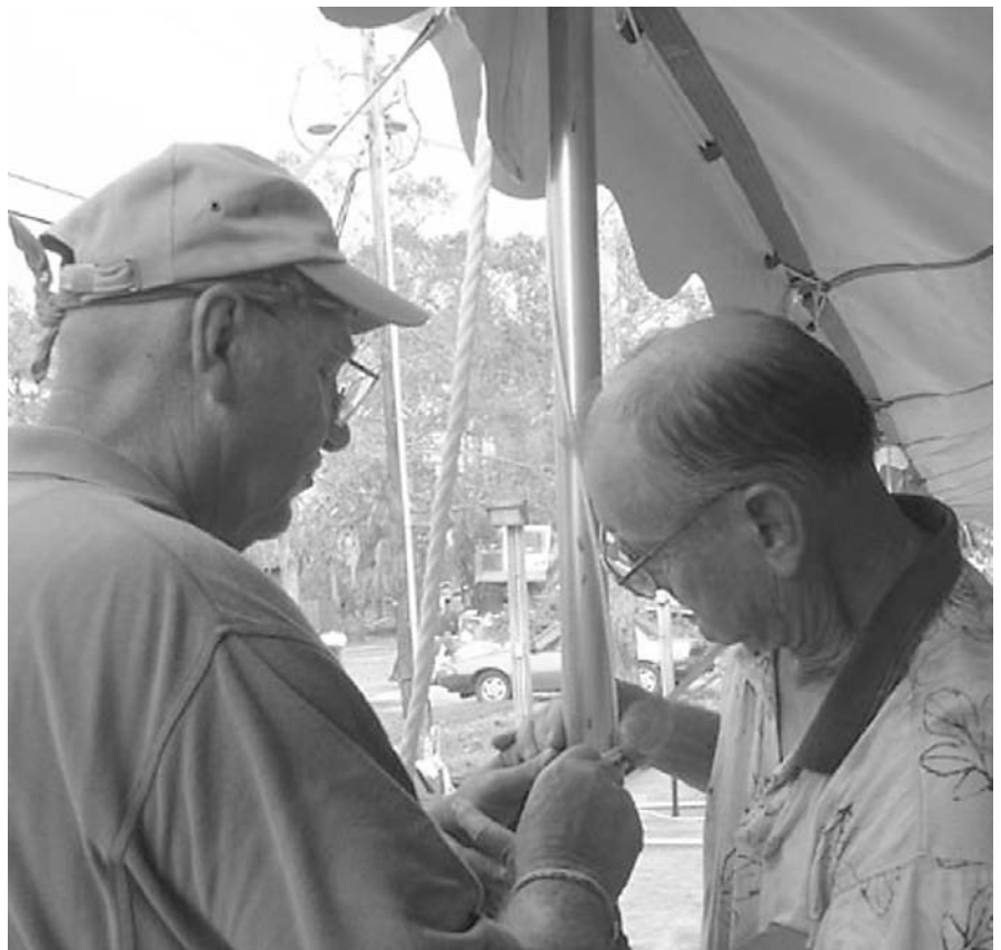
Tony Buesing (left) and Ernie Banner erect a 40-by-80-foot tent that will be used to store gifts-in-kind at Bethany Lutheran Church in Slidell, LA. Sue H. Poss photo
